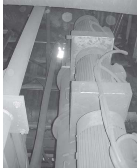
A 3 cell rotary reclamation plant.
